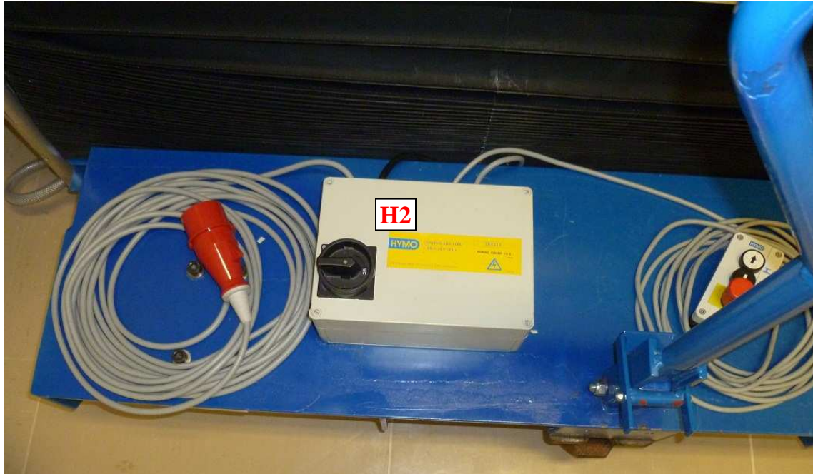
Fig.1: picture of the pre-existing external control box (labeled H2). Are also visible the cables connecting the box to the remote control and to the 380 Vac mains.
